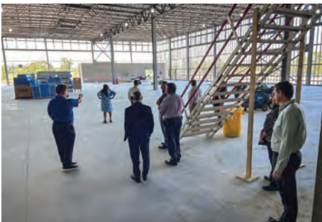
Select individuals received a sneak preview of the space under construction in August 2024.
